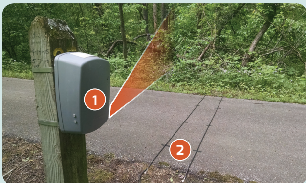
FIGURE 1 Counting equipment field installation
